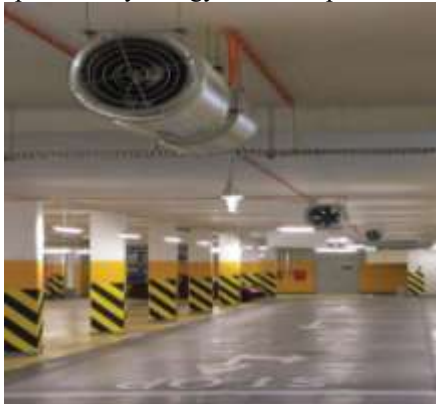
Figure 3 Ventilation in parkinglot
